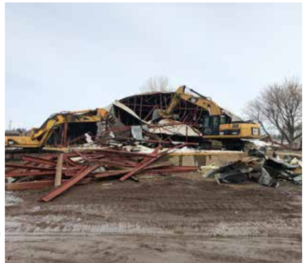
Use of NDR funds has allowed the City of Minot to acquire more than 100 properties to date that are needed to create greenway space for flood storage and floodwalls. A projected 74 properties remain to be purchased under this program.
